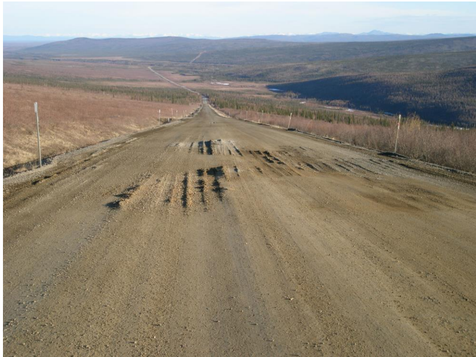
(a) Road conditions On May 12, 2010 (Before Treatment)
