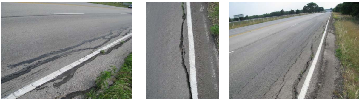
Figure 7. Sample distresses found on SH21 road before the rehabilitation plan
