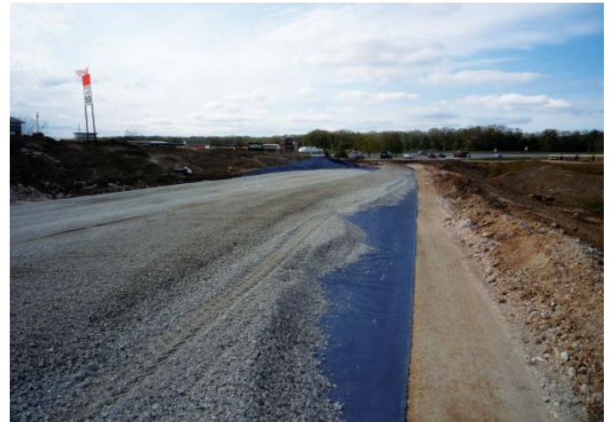
Almost 90,000 sq ft of geosynthetic material have been installed at the Daniel Boone Bridge.
