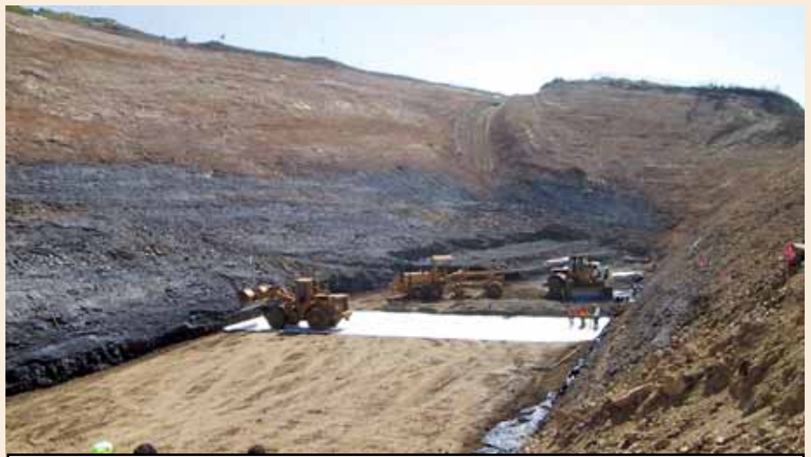
Photo 3. Numerous geotextiles and soil baskets provided vital internal support for the refilled hole.
