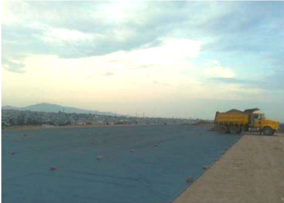
Image 1 – Mirafi® H2Ri Installed Parallel to Planned Traffic Flow Over a Prepared Subgrade
