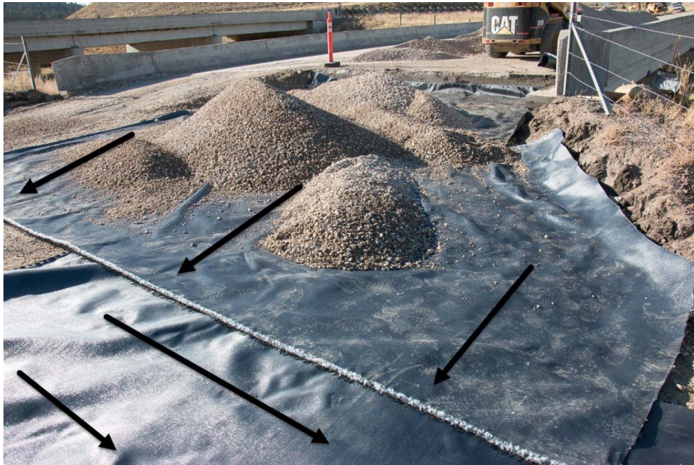
Image 5 - Bridge Approach, Routing Water Away from Structure.
